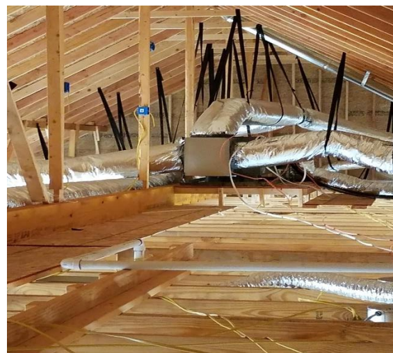
HVAC DUCT HANGERS
